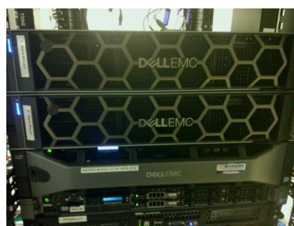
Figure 11 : Photos serveurs VMware DELL EMC
